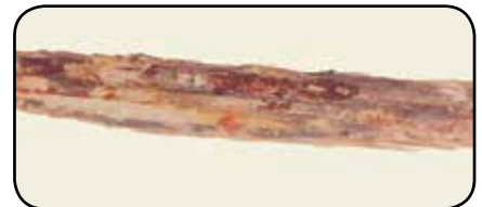
Close-up (25X) of UNPROTECTED scribe (scratch) showing pitting, metal loss & severe corrosion.
